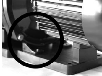
Regularly check the waterproofness! (A leak through a mechanical seal can cause important damages!)
